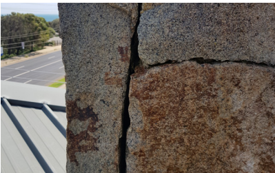
Stonework has unfilled joints, this allows water which strikes the stonewall during rain events to percolate to the back of the stone to the mortar/ adhesive bed. This water is able to track behind the stonework until it meets a breach or other discontinuity.
