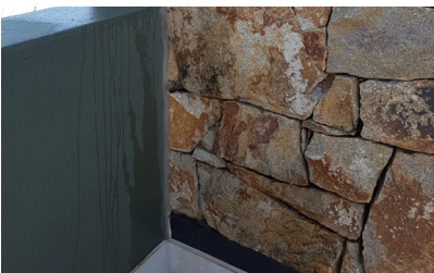
Area that has been isolated and is likely the primary area of water entry to the ceiling below.
