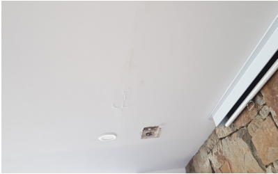
Areas showing where damage to ceiling plaster and redundant light fitting has occurred.
