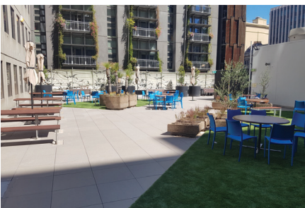
Finished installation featuring pavers and artificial turf on pedestals which can easily be lifted for maintenance inspection of the waterproof membrane and cleaning.
