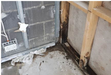
Water damage to timber framing from water travelling across floor slab.
