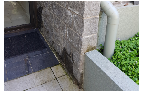
Water being drawn to internal floor slab due to poor building practices.
