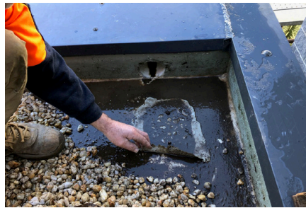
Blistering revealed on roof membrane.
